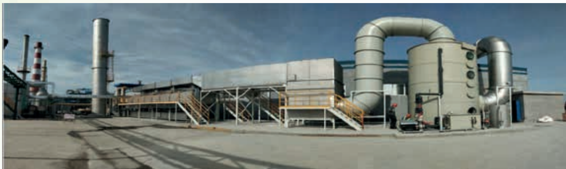
Figure 2 Flue Gas Ventilation and Dust Removal Facilities at Xiangshui New Universe 圖2響水新宇烟氣通風除塵設施
