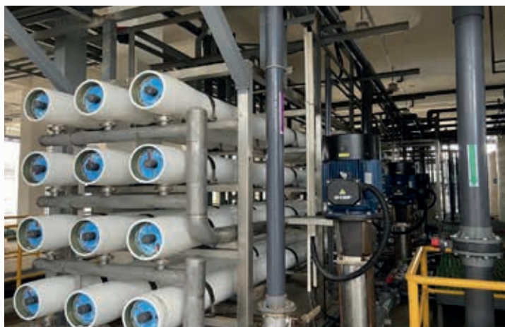
Figure 1 Water Recycling System at the Eco-plating Specialised Zone
