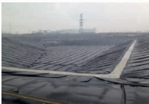
Figure 3 Anti – Seepage and Leakage Improvement Work at Yancheng NUHF 圖3鹽城新宇輝豐防滲防漏改造工程
