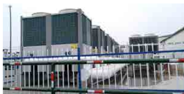
CSH Mine installed air-source heat pumps.
