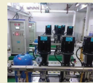
Variable-frequency non-negative pressure system in pump houses
