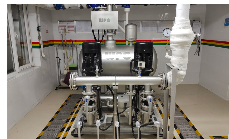
北京遠洋天地項目生活供水泵房系統 Domestic water supply pump system at Ocean Paradise (Beijing)
