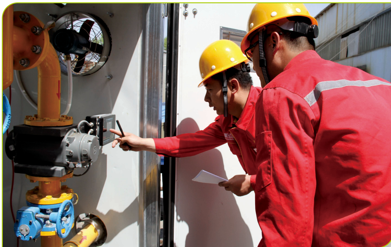
Regular Inspection of Work Equipment 定期設備檢查
