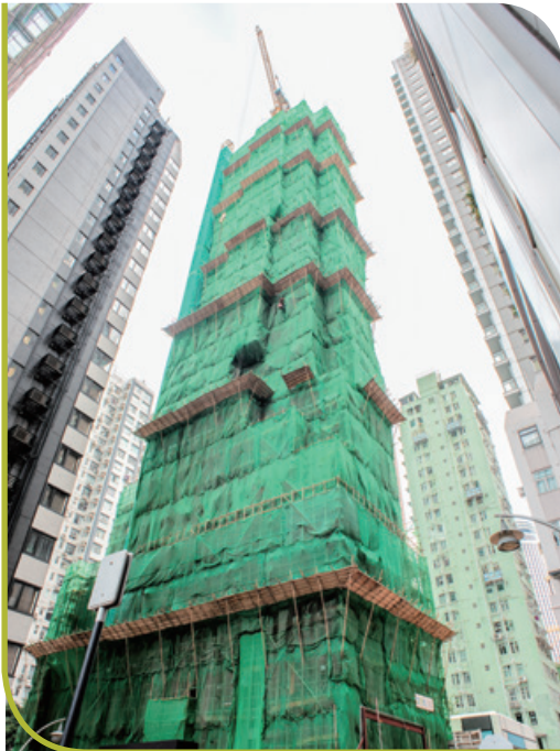
Residential redevelopment at No. 8 Star Street, Wan Chai (previously known as Nos. 21-31 Wing Fung Street, Wan Chai) 灣仔星街8號(前稱為灣仔永豐街21號至31號)之住宅重建項目
