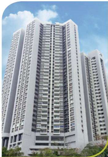
Building renovation works of Cavendish Heights (Block 1-7) at No. 33 Perkins Road, Jardine's Lookout 渣甸山白建時道33號嘉雲臺 (1-7座)樓宇之裝修工程
