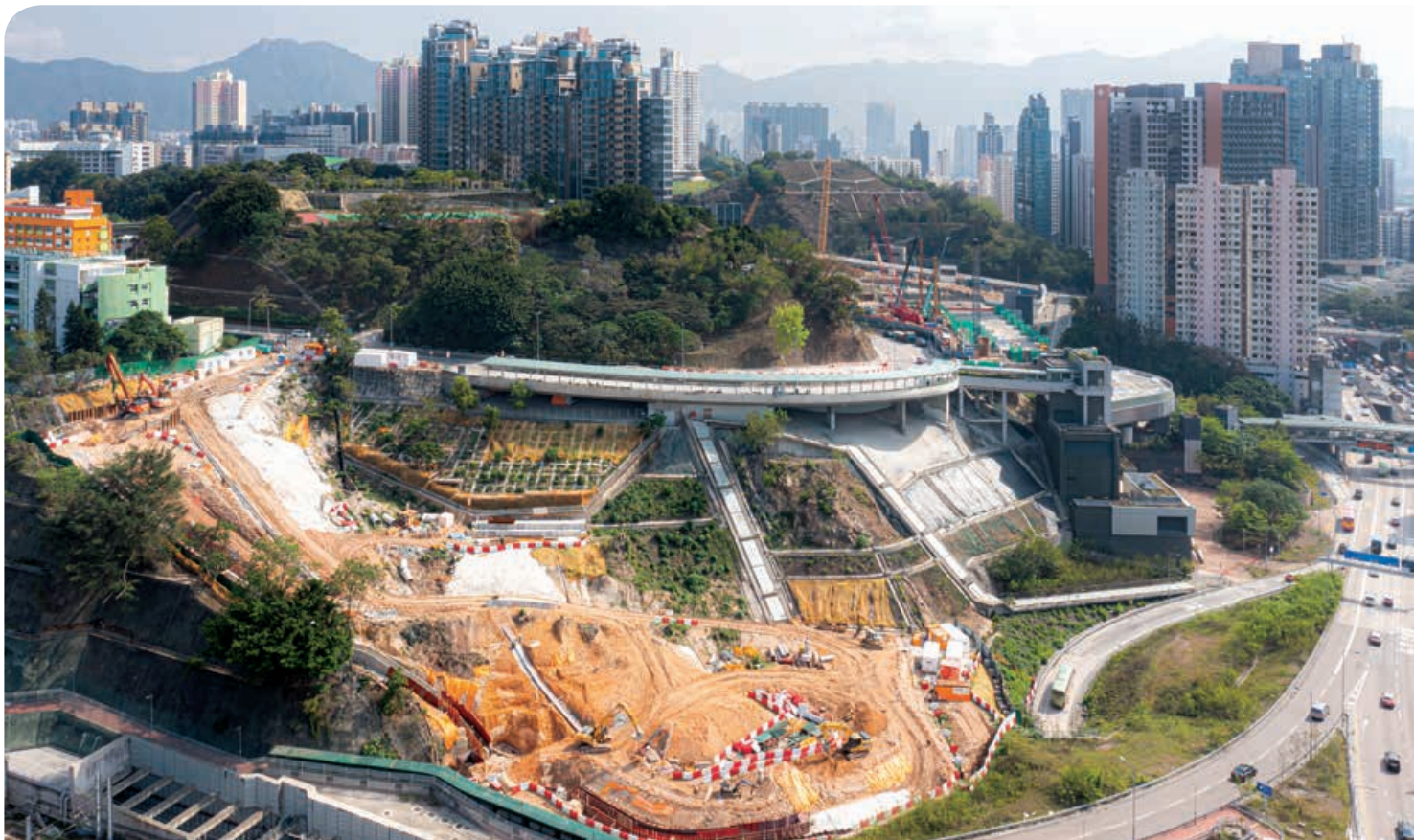
Site Formation and Foundation Works For Campus Expansion at Ho Man Tin Slope for the Hong Kong Polytechnic University 香港理工大學何文田斜坡校園擴建的地盤平整及地基工程
