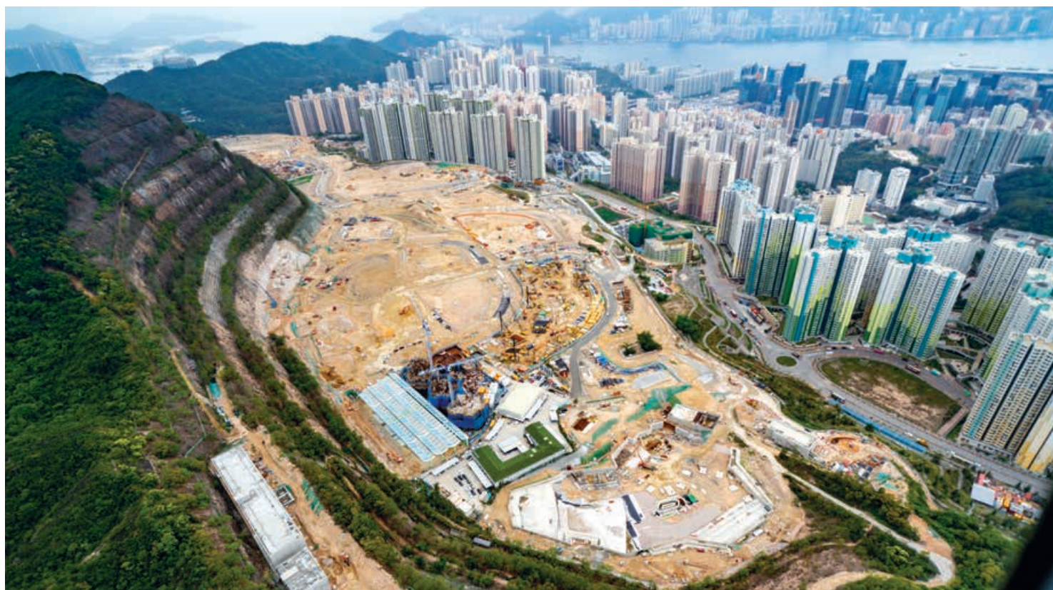
Site Formation and Infrastructure Works for Development of Anderson Road Quarry Site 安達臣道石礦場用地發展的土地平整及基礎建設工程
