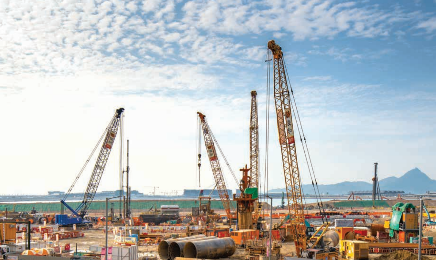
Foundation for Public Housing Development at Tung Chung Area 99 東涌99區公營房屋發展項目地基工程
