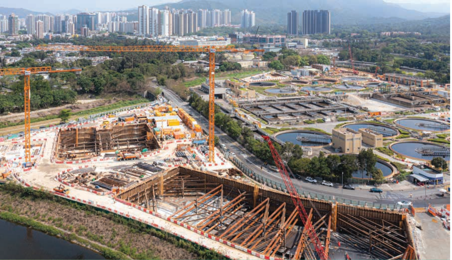
Shek Wu Hui Effluent Polishing Plant — Main Works Stage 1 — Civil Works for Sewage Treatment Facilities and Civil Works for Sludge Treatment Facilities and 132kV Primary Substation 石湖墟淨水設施 — 主體工程第一階段 — 污水處理設施的土木工程及污泥處理設施及 132kV 主變電站的土木工程
