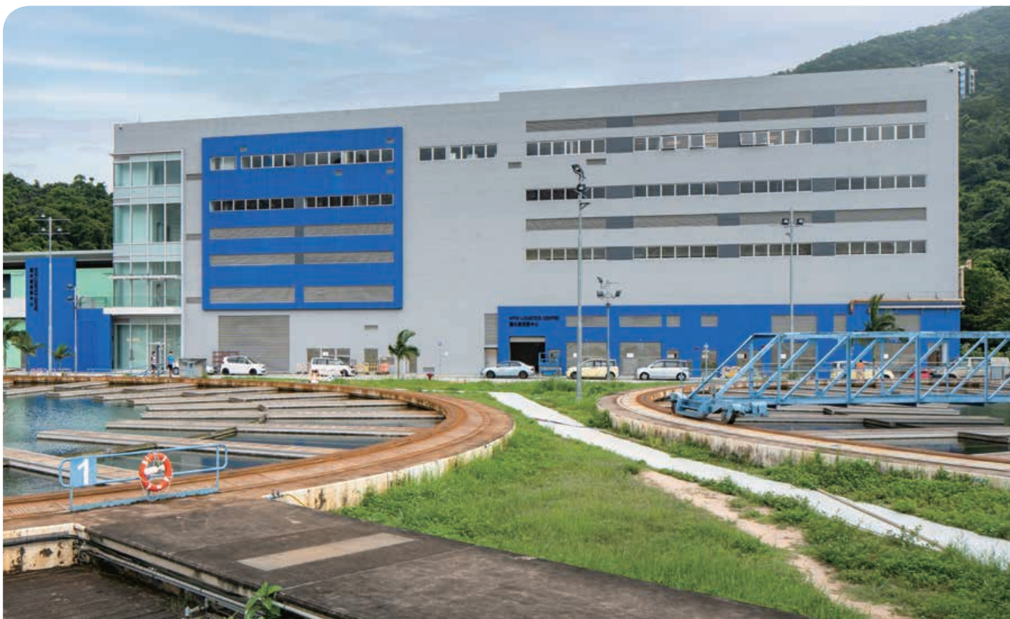
In-situ Reprovioning of Shatin Water Treatment Works (South Works) — Advance Works 沙田濾水廠原地重置工程(南廠) — 前期工程
