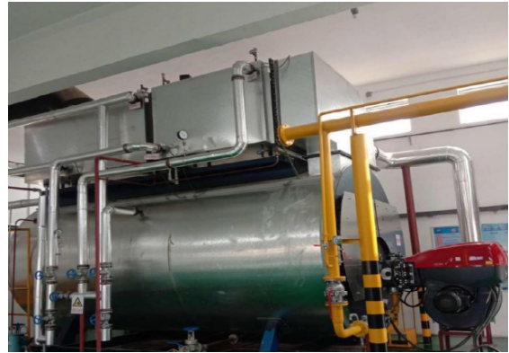
Boiler Heat Recovery 鍋爐餘熱回收設備
