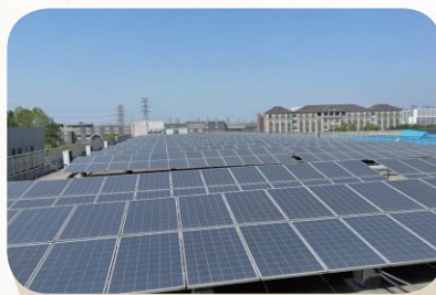
Photovoltaic power generating facility
