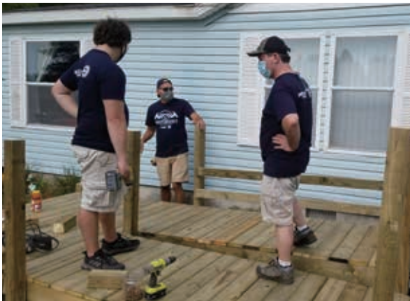
Nexteer volunteers build a handicap access ramp for people in need to allow them the ability to freely leave their home
