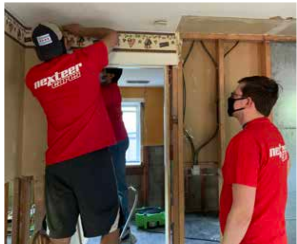
Nexteer volunteers helping to repair home affected by the flood for renovation
