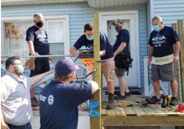
Nexteer volunteers build a handicap access ramp for people in need to allow them the ability to freely leave their home
