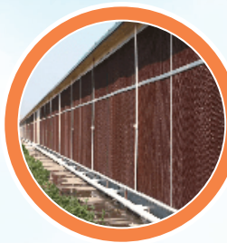
牛舍新風系統 Fresh Air System of the Cowshed
