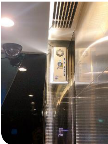
UV air purifiers in the lift
