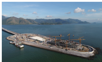
Eastern artificial island project of the Hong Kong-Zhuhai-Macao Bridge, a bridge-island-tunnel system
