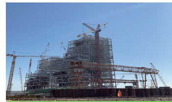
Yu County power plant in Wenchi Village, Niucun Town, Shanxi
