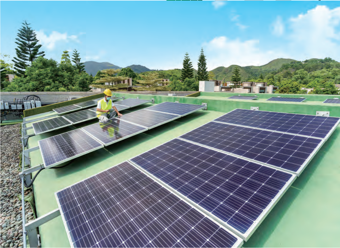
○ Energy-saving solar panels are installed in residential projects
