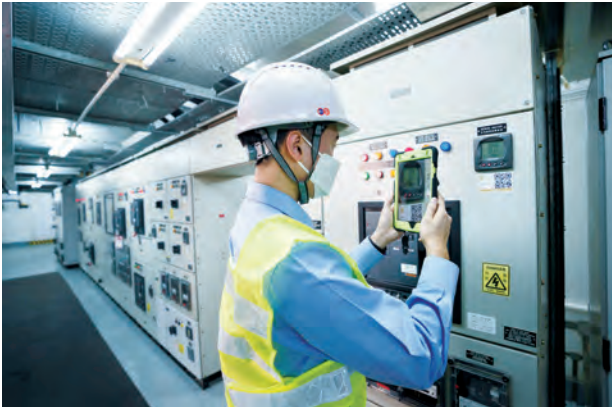
○ Engineers examine a facility's operations by scanning a QR code with a device installed with the IDEA system
