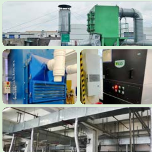
Exhaust air treatment facilities 廢氣處理設施
