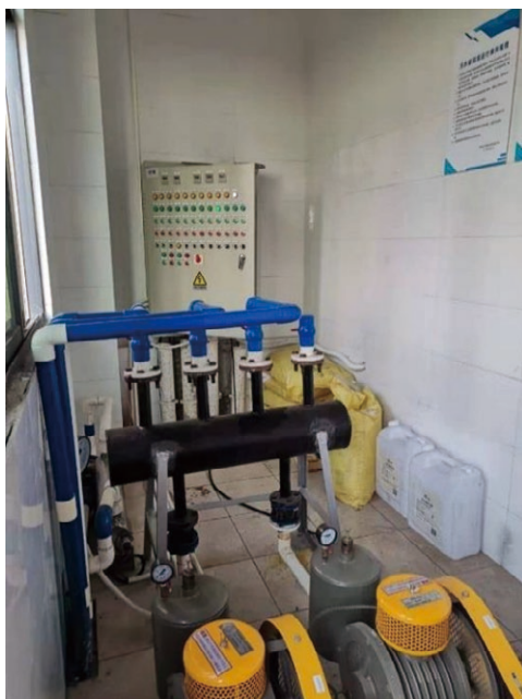
Hainan food factory - Wastewater treatment facility
