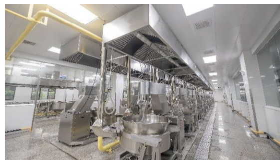
The highest degree of automation food production facility in new Hainan Carrianna food factory
