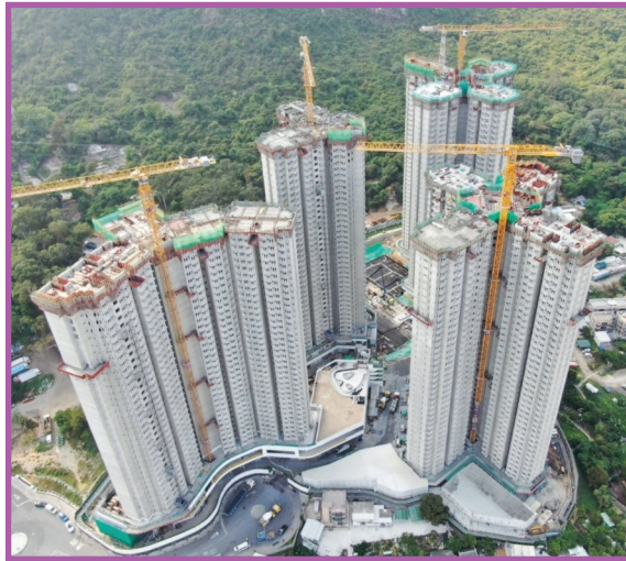
(One of our significant contracts – Construction of Public Housing Development at Tuen Mun Area 54 Site 1 & 1A) (我們的重要合約之一—屯門第54區第1及1A地盤的公共房屋發展建設)
