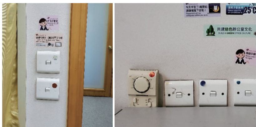
Energy saving slogan posted in office.
