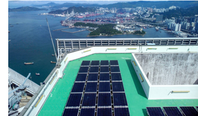
• More than 100 solar panels on ICC’s rooftop generate approximately 30,000 kWh per year and contribute to CLP’s Renewable Energy Feed-in Tariff scheme
