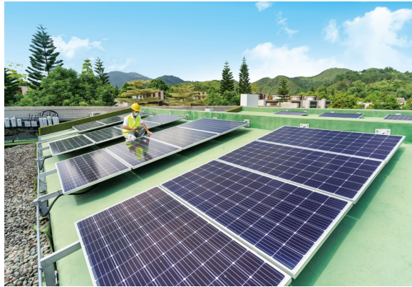
• Solar panels installed on the rooftops of buildings
