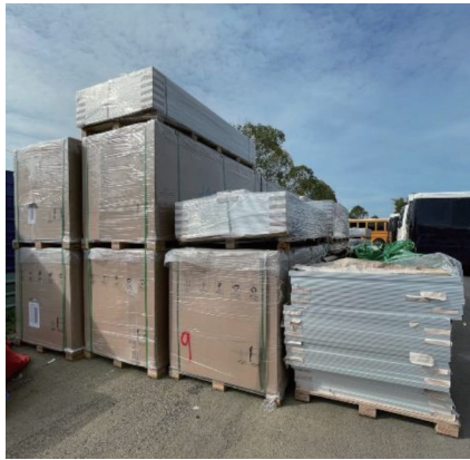
Preparation work for the installation of the Group's first solar photovoltaic system
