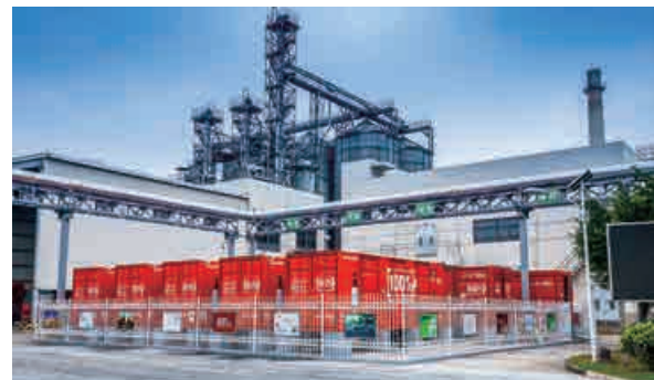
Foshan power storage system.
