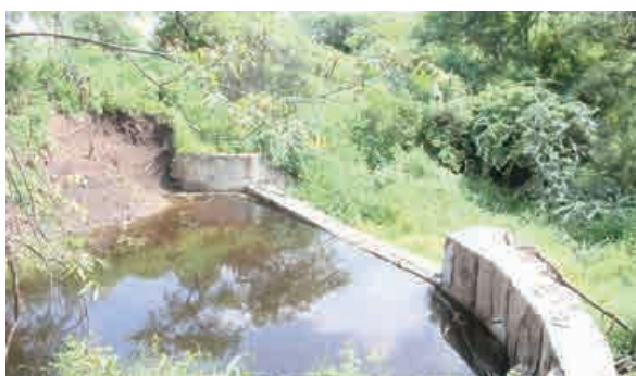
In the past ten years, we have constructed over 500 watershed structures across 13 villages in India.
