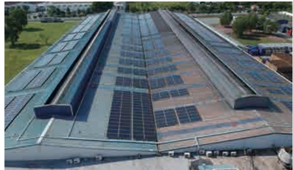
Two of our breweries in Vietnam entered the second phase of the solar project.
