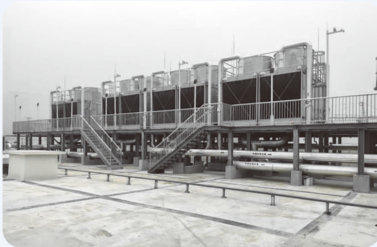
Cooling tower cluster of the data centre
