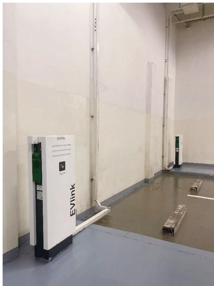
EV charging facilities at PCP Jakarta
