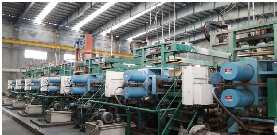
Sludge recycling equipment 污泥回收設備
