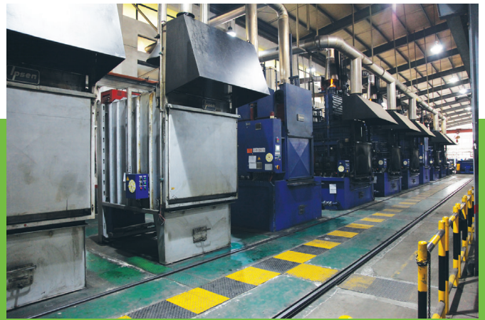
中國廣東省河源廠的多用途熱處理爐 Multi-purpose heat treatment furnaces at Heyuan factory, Guangdong Province, China
