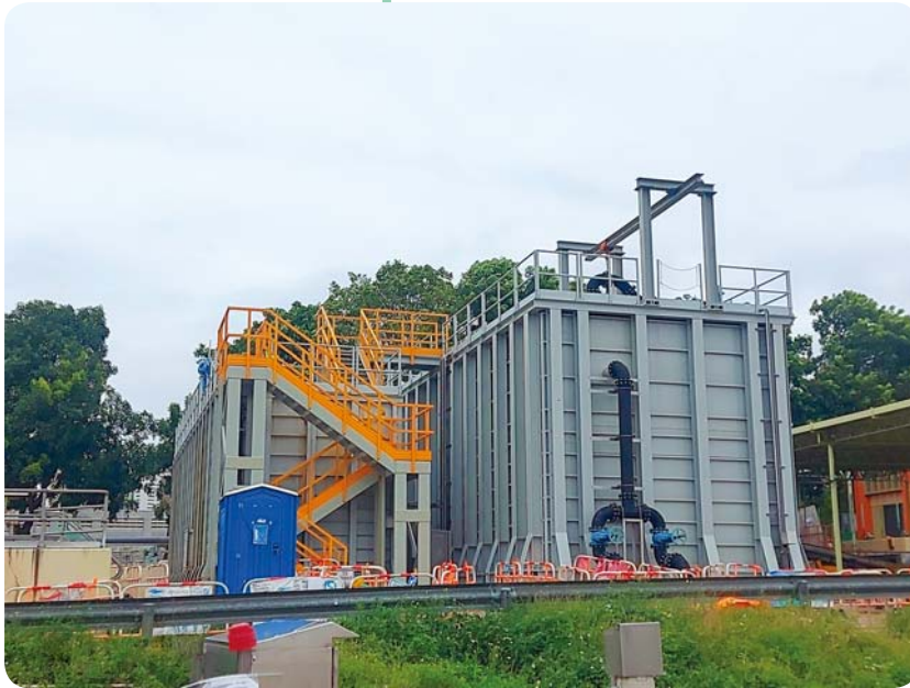
Shek Wu Hui Effluent Polishing Plant – Main Works Stage 1 – E&M Works for Sewage Treatment Facilities
