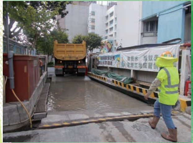
Provide vehicle washing facilities at site exits to wash away dusty materials from vehicle wheels before they leave the site 在工地出口處提供洗車設施，以便在車離開前清洗車輪上易生塵埃物料
