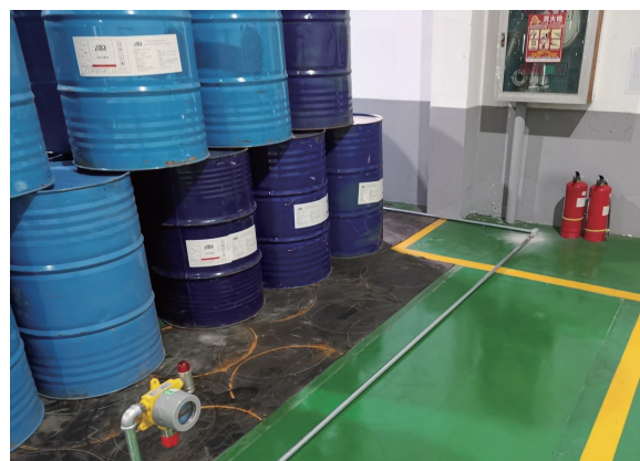
Safety alarms and fire fighting equipment
