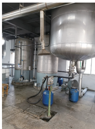
Active-carbon gas absorption system
