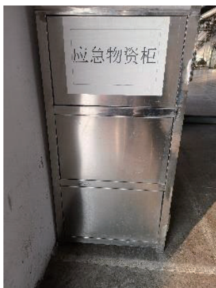
Emergency supplies cabinet
