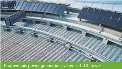
Photovoltaic power generation system at CITIC Tower
