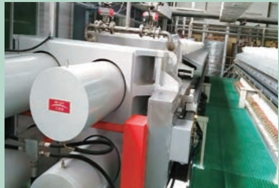
Oil-pressure dehydration equipment
