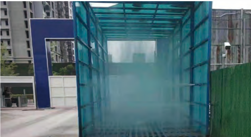
Car cleaning equipment is installed at the entrance of the construction site
