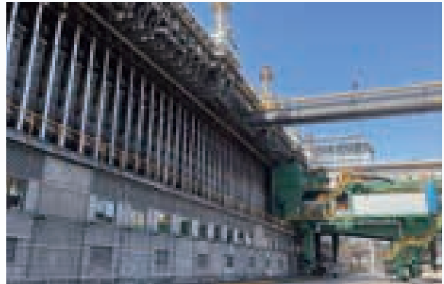
Coking furnaces with height of 7.65 metres
