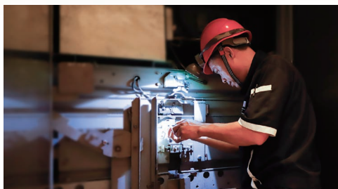
電梯服務 Elevator Services
