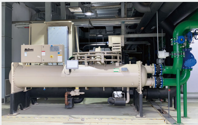
500RT inverter centrifugal chiller
