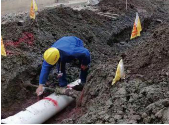
Photo: An on-site supervisor paints a warning mark and puts up warning flags
