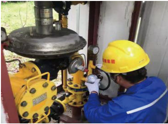
Photo: An inspector inspects the pressure regulating equipment
