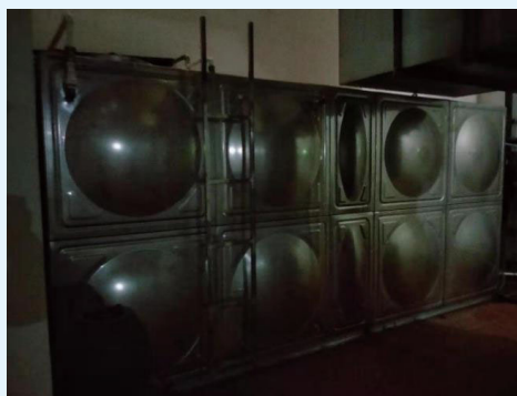
Photo: Installation of Additional Hot Water Storage Tanks
