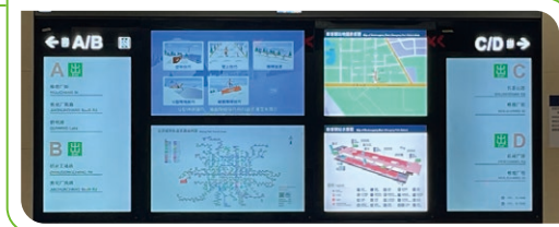
PIS and e-directory signs at ground level
