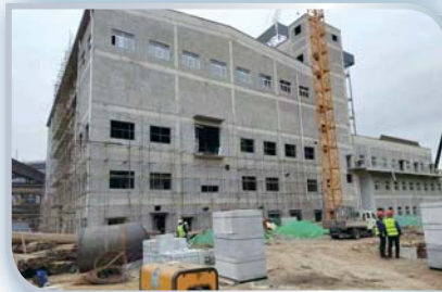
Jinxi Limited builds a supercritical gas electricity generation module 津西鋼鐵新建一座超臨界煤氣發電機組
