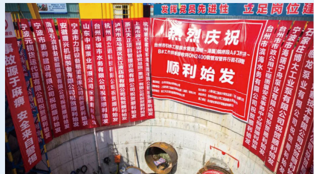
Taizhou Water Diversion Project – Pipe jacking operation for raw water transmission successfully completed
