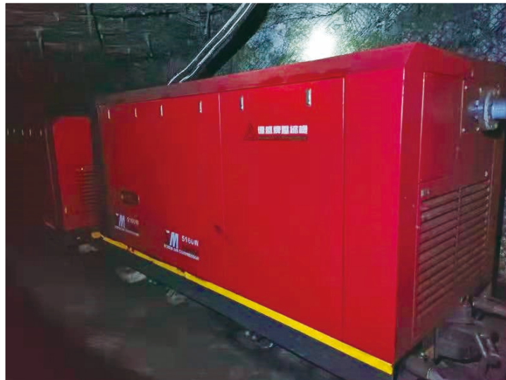
Picture: Nitrogen Generation System Device in Mine Panel at Zhaiyadi Coal Mine
