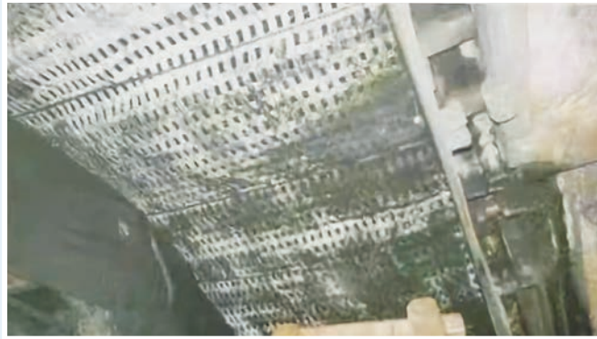
Picture: On-site Arrangement of Polyester Fiber Plastic Mesh at Xingwu Coal Mine
