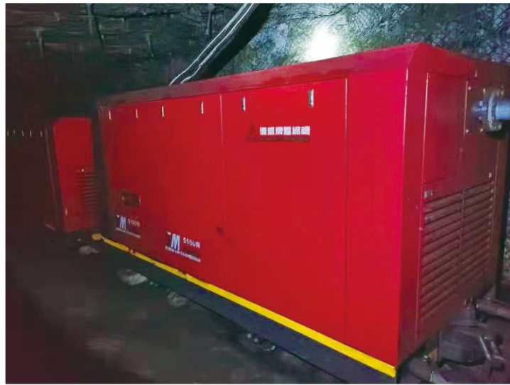
Picture: Nitrogen Generation System Device in Mine Panel at Zhaiyadi Coal Mine
