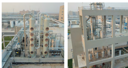
Solvent recovery plant
