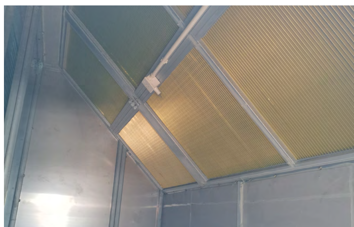
Heat recovery unit in the air-conditioning system (plate-fin heat exchanger)
