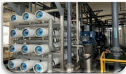
Figure 1 Water Recycling System at the Eco-Plating Specialised Zone
