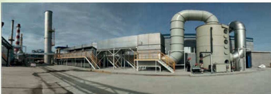
Figure 3 Flue Gas Ventilation and Dust Removal Facilities at Xiangshui New Universe
