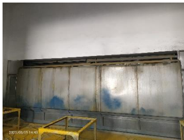
Water Curtain System for collection of spray paint exhaust
