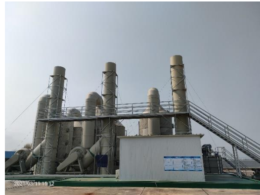
Acidic Mist Exhaust Treatment Facilities
