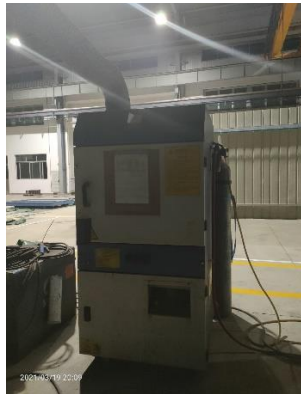
Movable Welding Smoke Treatment Facilities
