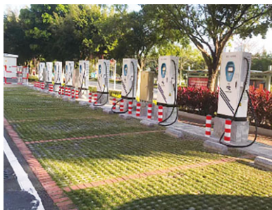
New Energy Vehicle Charging Piles
