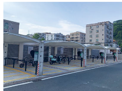
Electric Bike Charging Piles
