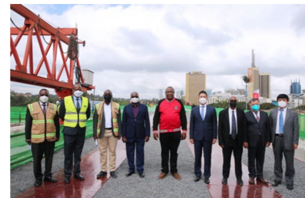
肯尼亚总统乌胡鲁·肯雅塔参加内罗毕快速路主线架梁贯通仪式 Kenyan President Uhuru Kenyatta presided over the laying of the last girders of the Nairobi Expressway
