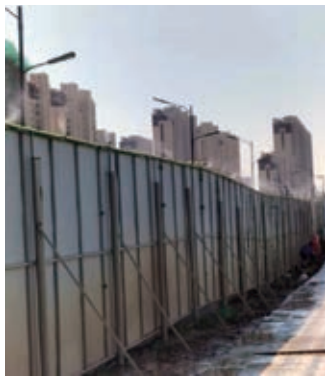
Spray at the end of the enclosure 圍牆端部佈置噴淋
