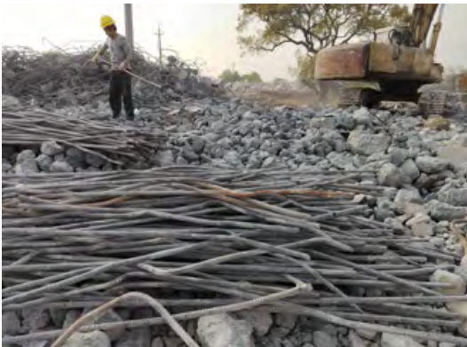
Dismantling temporary concrete bracing to recycle steel bar and concrete fragments in Westlake 66, Hangzhou
