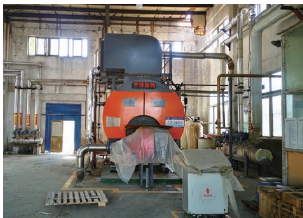
Natural gas boiler
