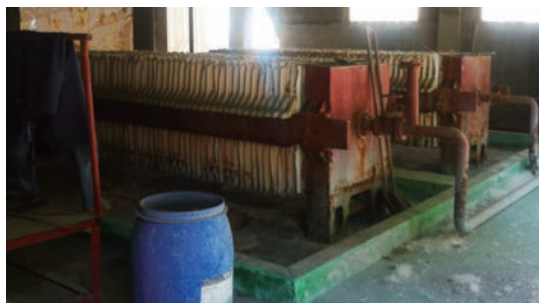
Sludge treatment filter press
