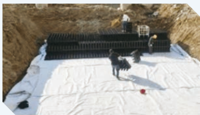
Rainwater recycling system
