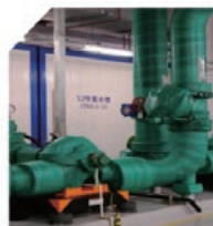
Ice storage equipment
