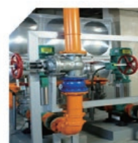
Reclaimed water treatment equipment
