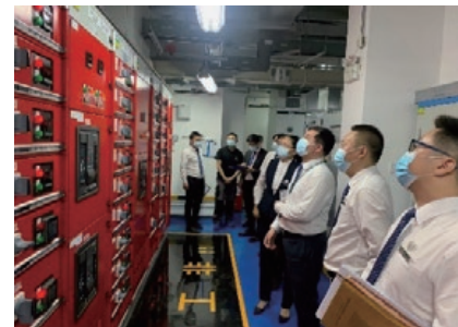
Guidance on visualization standards for engineering equipment rooms
