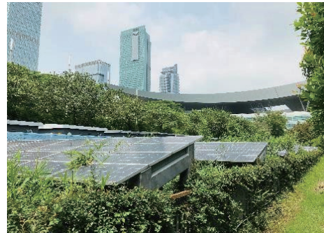
Solar retrofitting of underground parking lot
