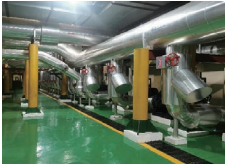
Transformation of the cold storage of air conditioning system
