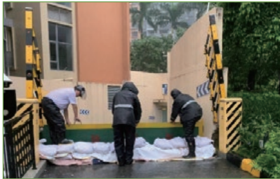
💧 Flood control sandbag dam for underground garage
